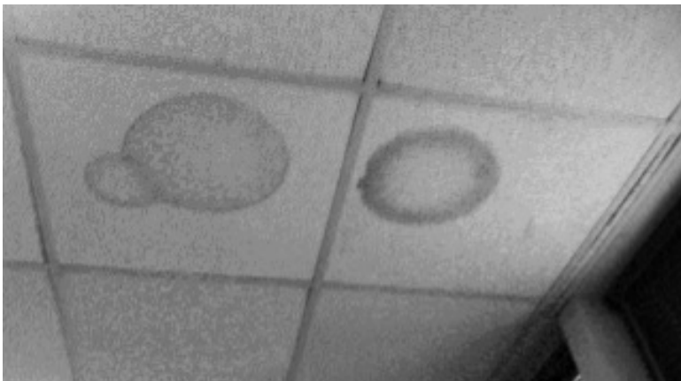
Figure 2: A photo of brown stains on ceiling tiles that reveal water damage that grew worse over time.
